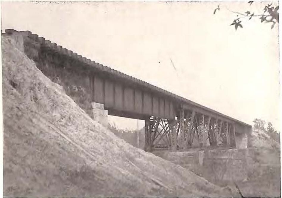
STEEL BRIDGE NEAR MANCHESTER, N. C., ON LINE OF ATLANTIC COAST LINE R. R.
