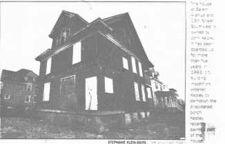
This house at Salem and 13th Street, South-west is owned by John Kape. It has been boarded up for more than five years. In 1993, city building inspectors ordered Kape to demolish the dilapidated porch. Kape recently painted part of the house.
