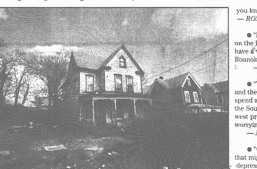
A Gilmer Avenue Northeast house, in one family for more than 50 years, is now vacant and condemned, its yard strewn with litter.
