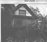
This vacant house on Marshall Avenue Southwest is one of the city's three best street numbers. A fourth number, 907, is on a notice from the building inspector that declares the structure unsafe.
