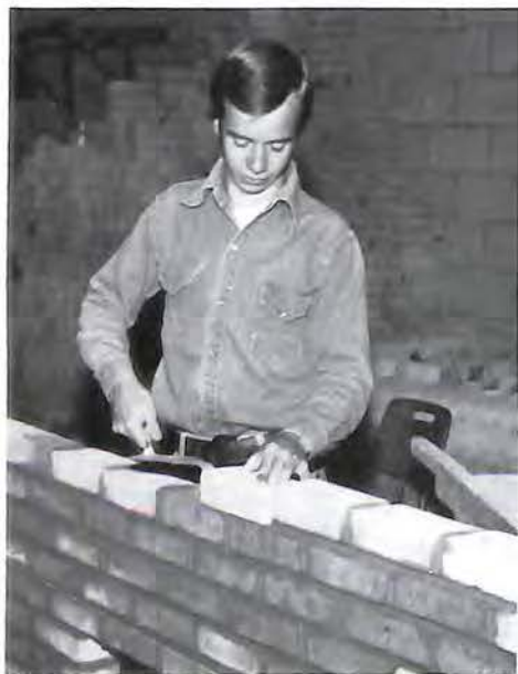
Mastering the fine art of masonry, Ralph Furrow carefully lays the bricks.
