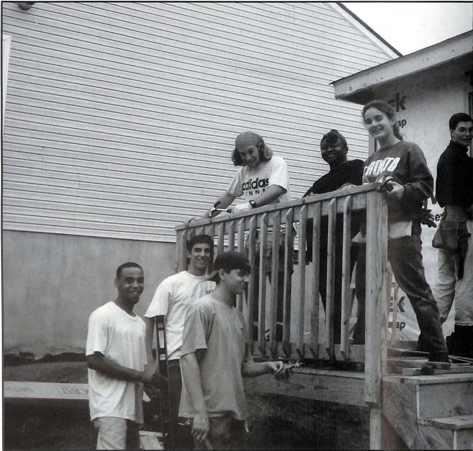
Juniors Matt Spetzler, Dan Spurlock, Brent Stover, and Emmy Spencer help out the Key Club in their Habitat for Humanity project. Members helped to construct a house with other volunteers from around the valley. "I really enjoyed working on Habitat for Humanity because I feel that it is a very worthwhile charity," said Emmy. "It didn't seem like a lot of work because I was with my friends."
