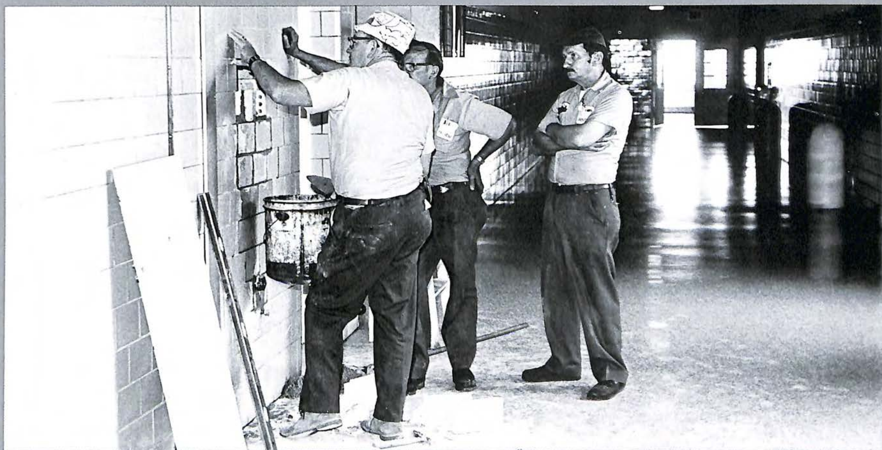
COLD WATER AT LAST Mr. Byron Poag, Mr. Ben Tatum and Mr. Jack Lucado from the Roanoke County Maintenance Department lay tiles to install a new water cooler-type fountain. The SCA and the senior class each gave one much-needed fountain as a gift.
