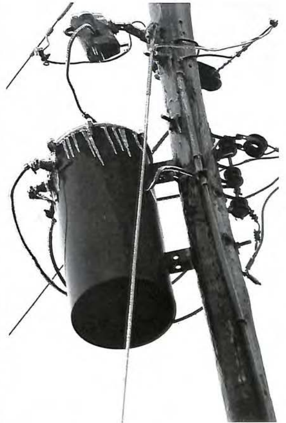
TRANSFORMERS Power lines snapped, transformers popped and fourteen thousand customers in the Roanoke Valley found themselves in cold, damp darkness. APCO worked for two weeks to get the lights back on around the valley.
