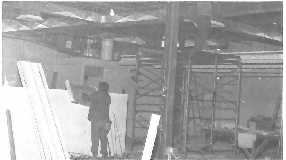
SHOWING RESULTS . . . The construction workers labor hard to complete the new extension to 'C' hall. The sights, sounds, and smells of construction became familiar to the students.
